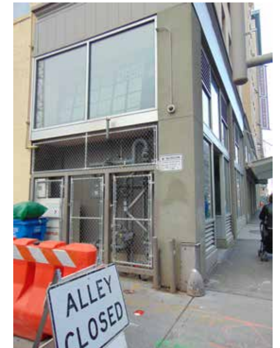
THE PLYMOUTH - UTILITY METER
