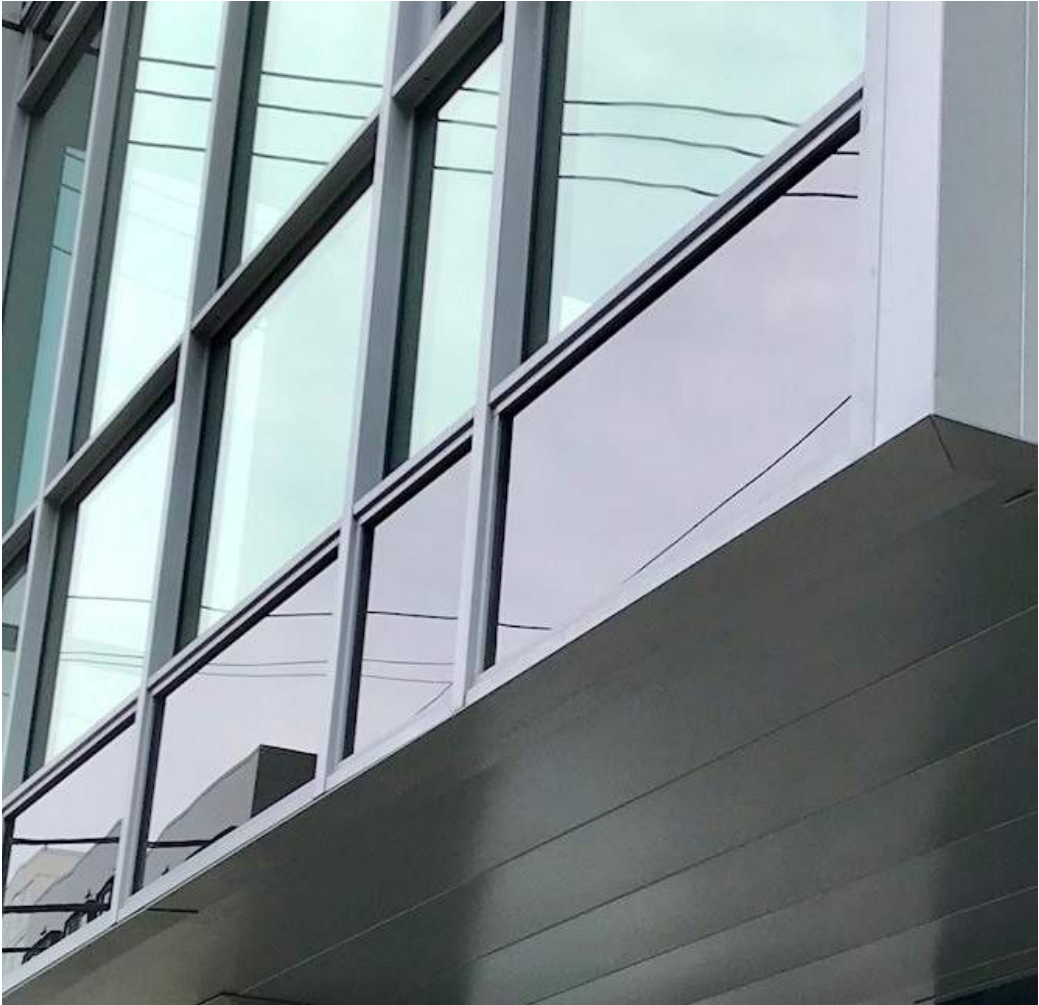
SIMILAR SOFFIT CONDITION
