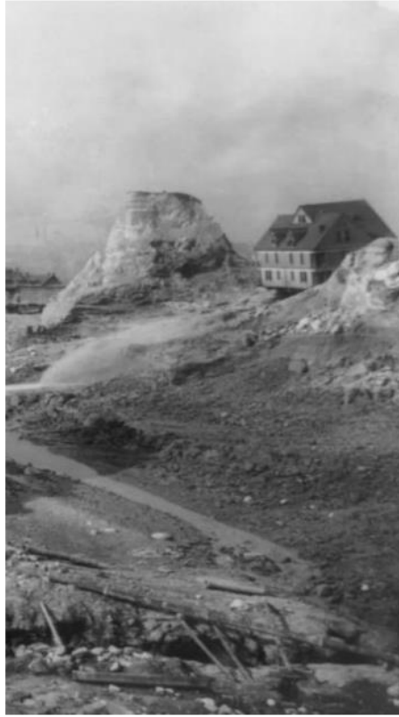
SEATTLE REGRAIDING INCLUDING SPITE MOUND AND DENNY RE-GRADE (SHOWN), IN PHASES, 1902-11 AND 1929-30
